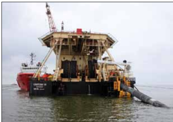
The first 28-kilometre pipeline segment in German waters was completed in mid-August, then construction continued on the second string.
