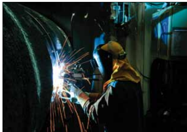
Pipes are welded into a double-joint segment on the Castoro Dieci in German waters. These double-joint segments will later be connected to the main pipeline.
