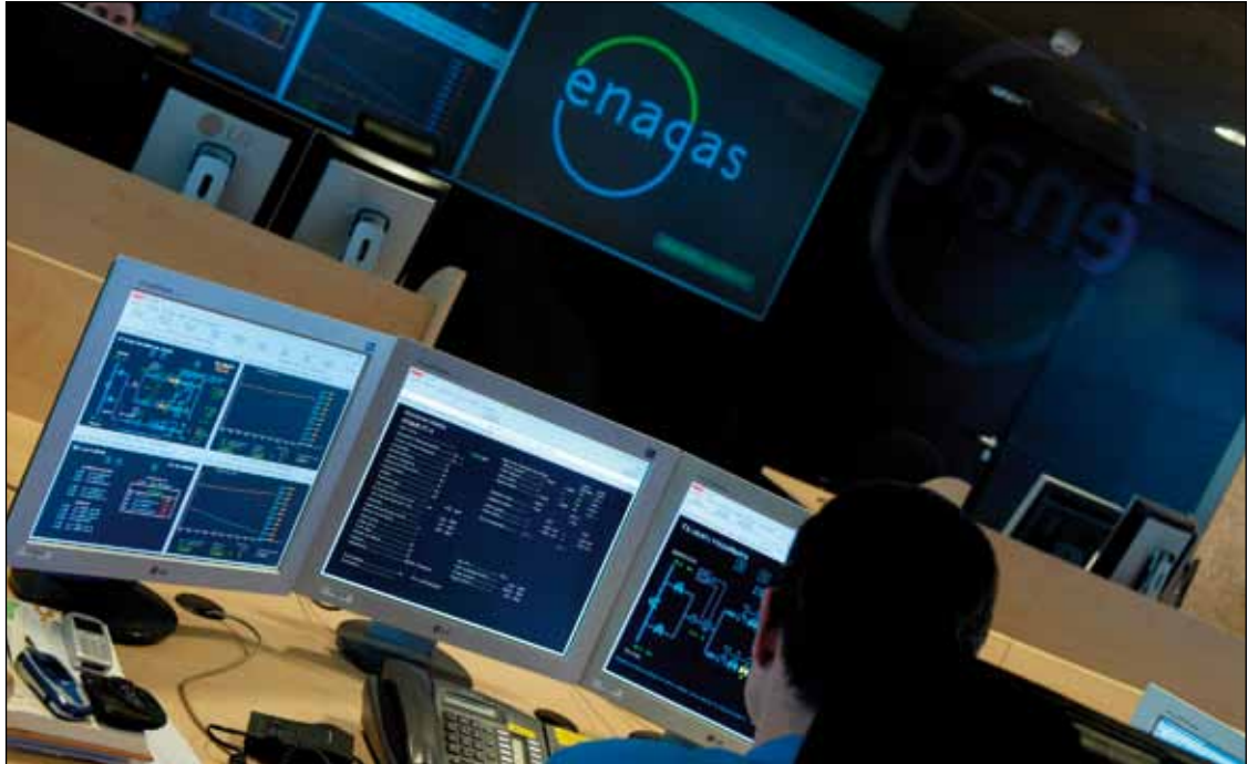
Enagás uses computer simulation, planning and other tools to run the gas pipeline network from its main control centre in Madrid.
